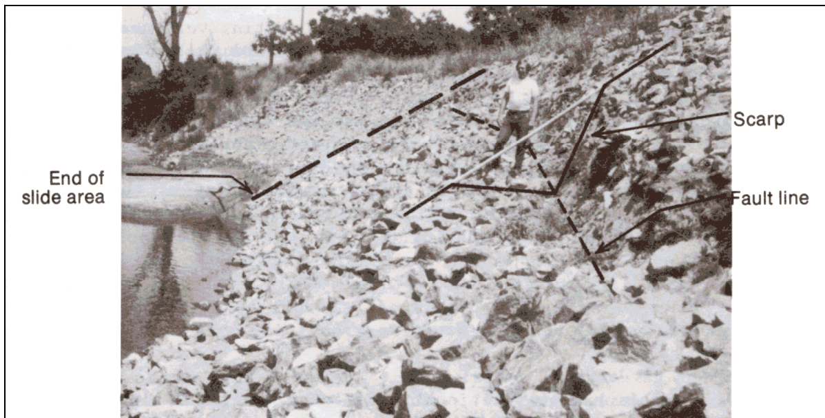
Figure 5.11. Riprap on Cosumnes River at Site 2 near Sloughhouse, CA, looking downstream, showing translational slide failure (photographed May 31, 1983) (Blodgett & McConaughy 1986).
