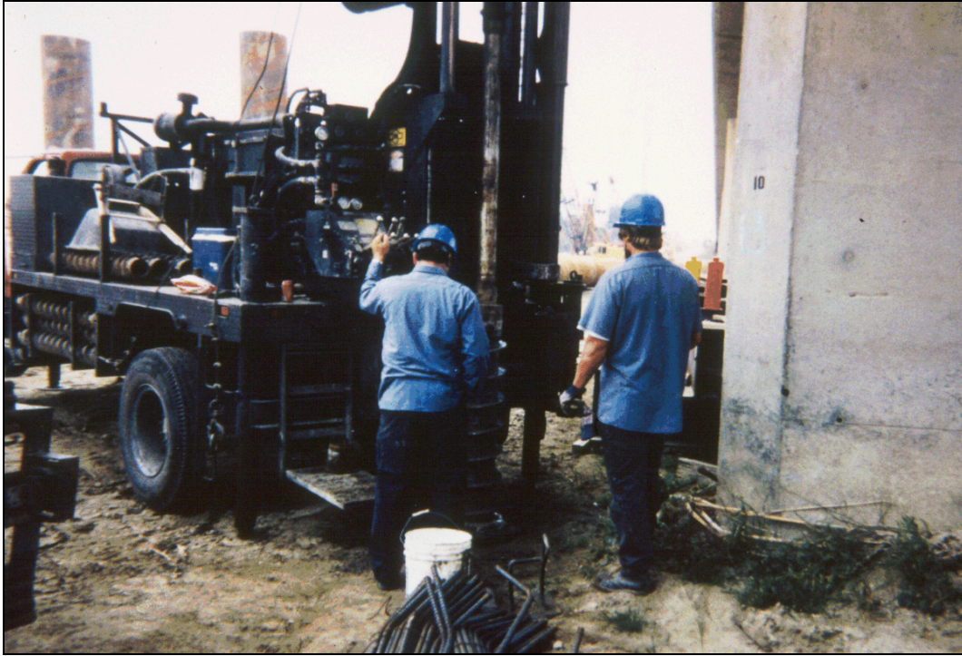
Figure 9.29. CALTRANS drilling with hollow stem auger for installation of float out devices at Salinas River Bridge (Highway 101) near Soledad, CA.
