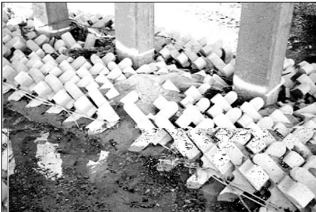
Figure 5.24. Installation of A-Jacks® modular units installed by Kentucky DOT for pier scour protection.
