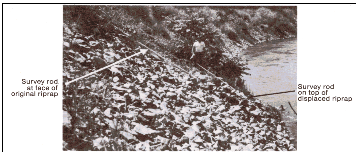
Figure 5.13. Riprap on Consumnes River at Site 3 near Sloughhouse, CA, looking downstream, showing modified slump failure (photographed May 31, 1983) (Blodgett & McConaughy 1986).
