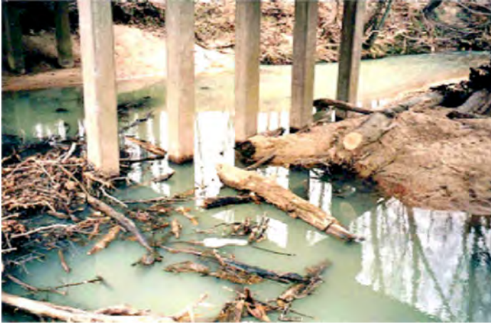
Figure 19.5a. Scour hole debris at Bridge 133, Graves County, KY
