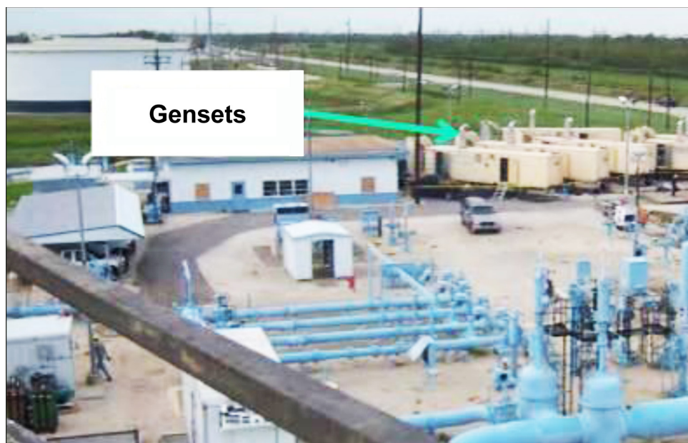
Figure 12: Colonial's Portable Generators
