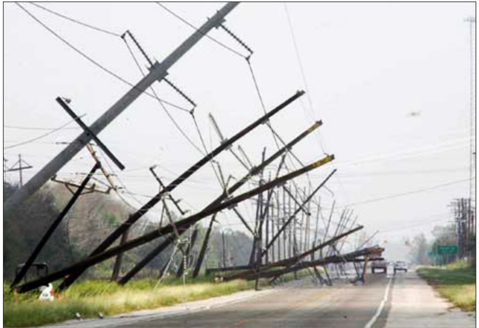
Figure 10: Fallen Transmission Lines after Hurricane Rita
