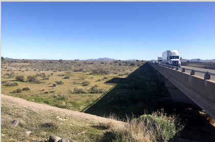
Source: GAO analysis of information from ADOT. Photo: GAO. | GAO-21-436
