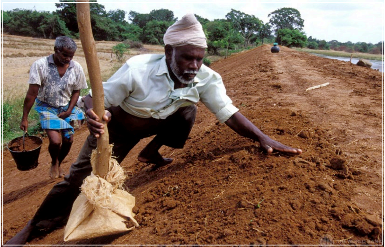
Two men repair breached sections of embankment in Sri Lanka. Photo: Dominic Sansoni/World Bank
