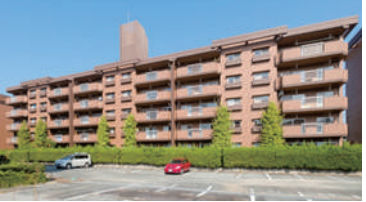
<The fourth building had the largest inclination as pilings were damaged to cause inclination>
