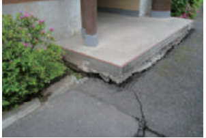
<Subsidence caused liquefaction>
