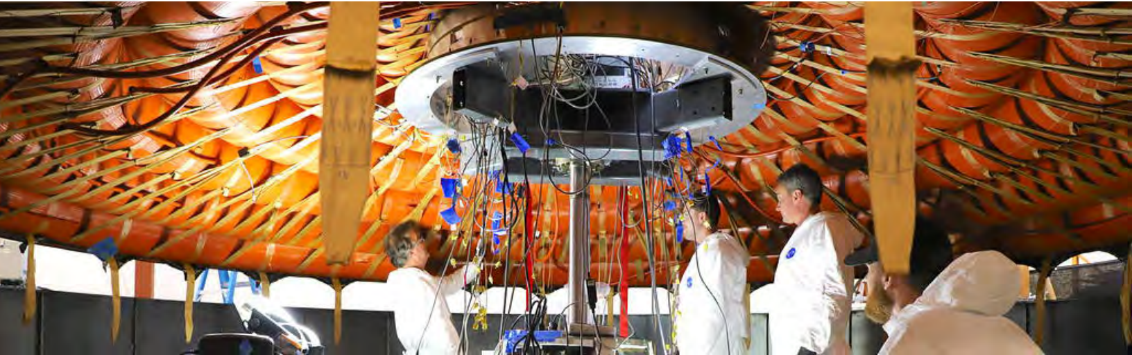
Engineers prepare for the flexible heat shield installation on the inflatable structure. The view is from bottom side, heat shield is on top. The gold straps hanging from the black triangles will be attached to the inflatable structure strapping and tensioned. Credit: NASA's Langley Research Center.
