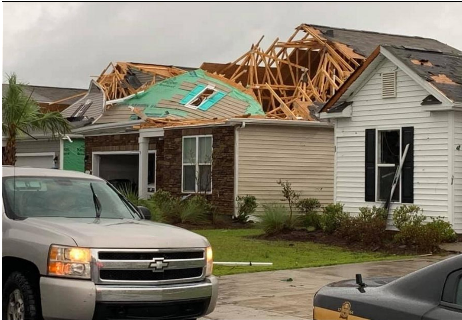
Figure 11. Roof damage to homes in Brunswick County, North Carolina, caused by an EF2 tornado on 5 September 2019. Picture courtesy of Brunswick County Sheriff's Office.
