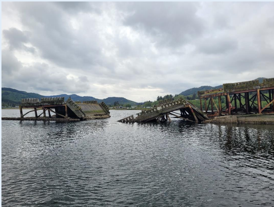
The I-90 floating bridge segment, which will be removed as part of the NOAA Marine Debris Program's BIL grant award to the National Marine Sanctuary Foundation. Photo credit: NOAA.
