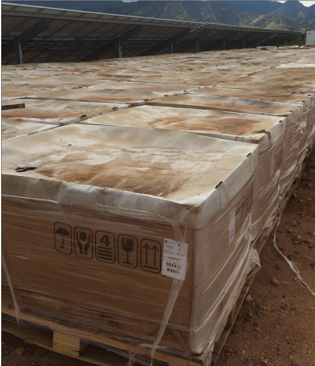
Figure 16. Failure to follow product box handling and storage requirements can cause damage when moved and void a warranty. The umbrella symbol on this box indicates it should be kept dry and the box might fail when picked up with a forklift. Photo by Andy Walker, NREL
