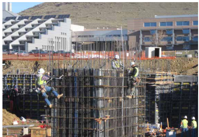
NREL’s Research Support Facilities (RSF) under construction. Photo by Carl Cox, NREL 16282
