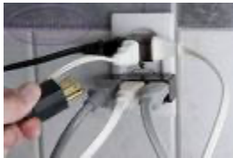
No - Overloaded circuit!
