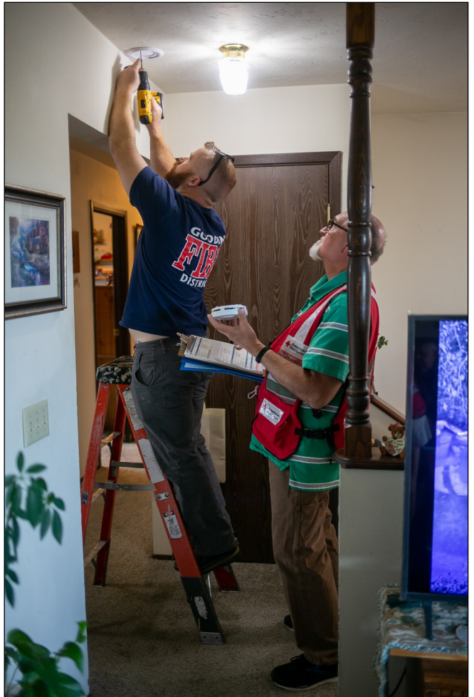
Dennis Becker, green shirt, teams up with a Gooding firefighter to install a smoke alarm in an Idaho home. Red Cross and its partners installed 370 free smoke alarms during the multi-state Sound the Alarm program.
