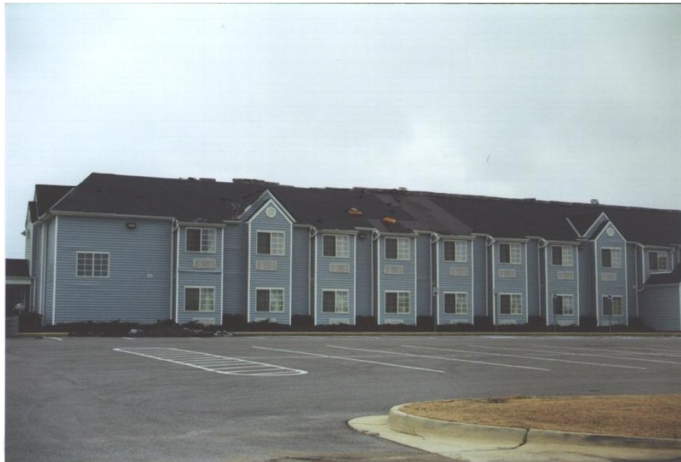
ACT: DOD 2: Loss of roof covering (<20%)
