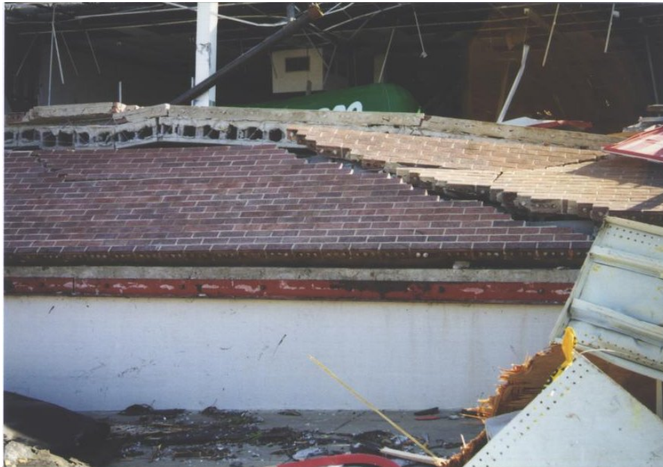
WHB: DOD 6: Collapse of non-bearing exterior wall
