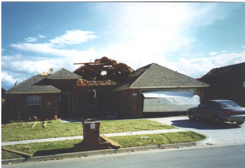
FR12: DOD 4: Uplift of roof deck and loss of roof covering (>20%); garage door collapses outward
