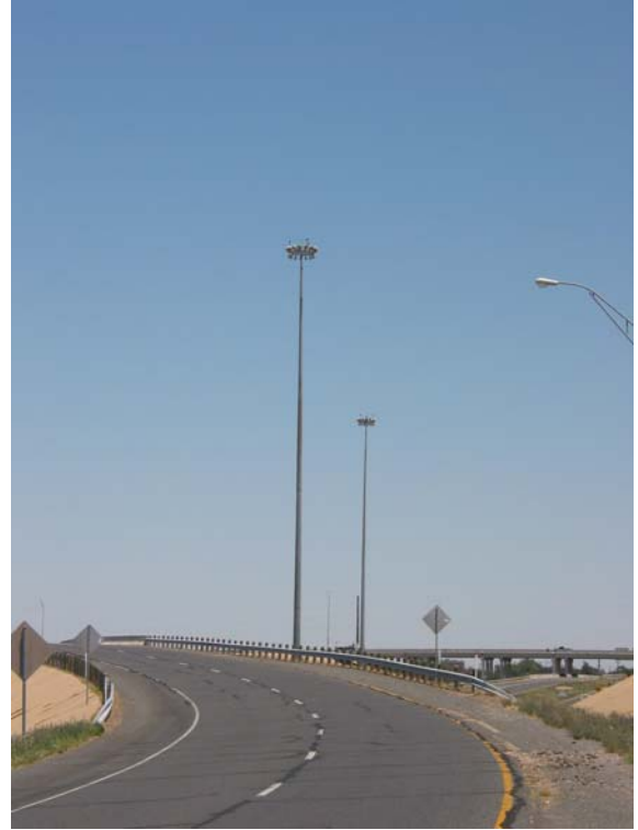
FSP: Luminary Poles
