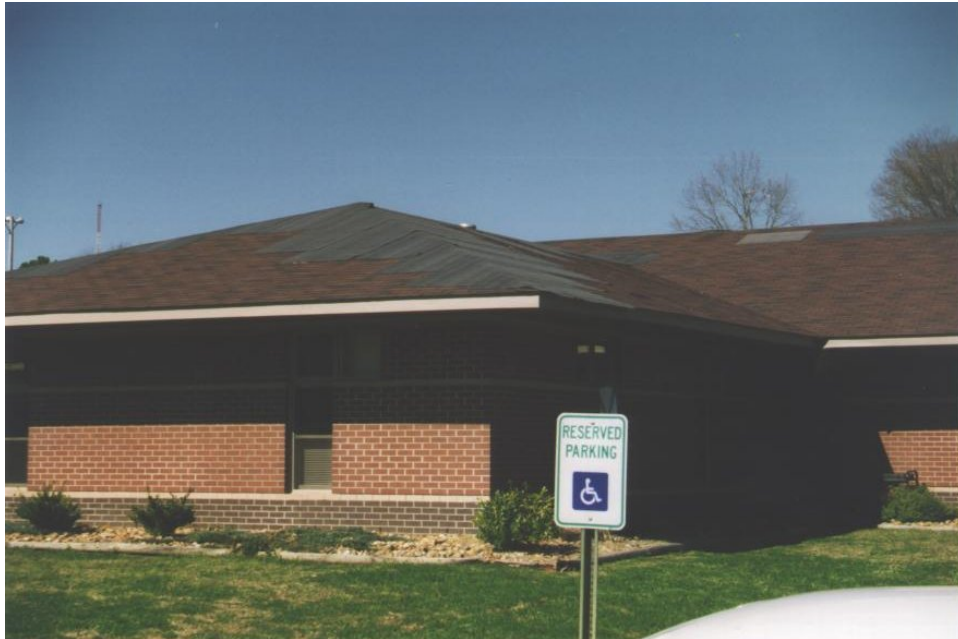
FR12: DOD 2: Loss of roof covering (<20%)
