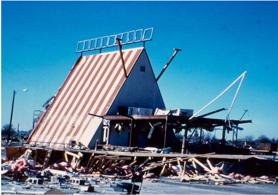
SRB: DOD 5: Canopies and covered walkways destroyed
