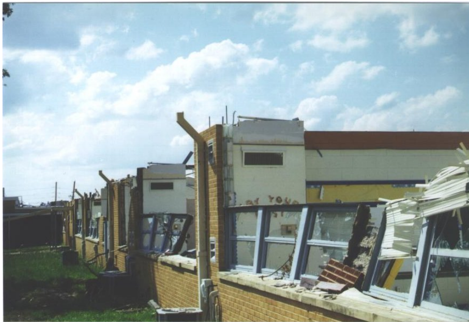
ES: DOD 7: Uplift of entire roof structure
