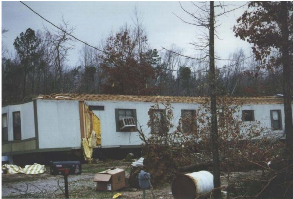
MHDW: DOD 5: Uplift of roof deck and loss of significant roof covering material (>20%)
