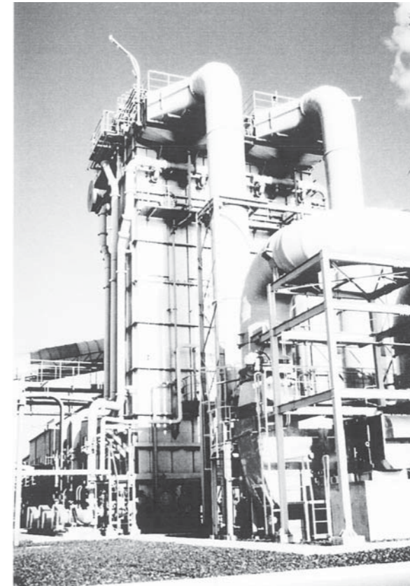
図2 石灰石膏法設備 Fig.2 Photo of desulfurization plant (Gypsum process)
