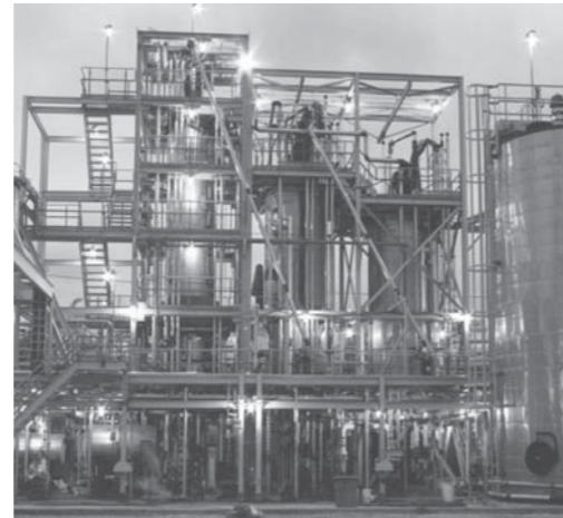
図8 設備外観 Fig.8 Photo of PDCB production plant
