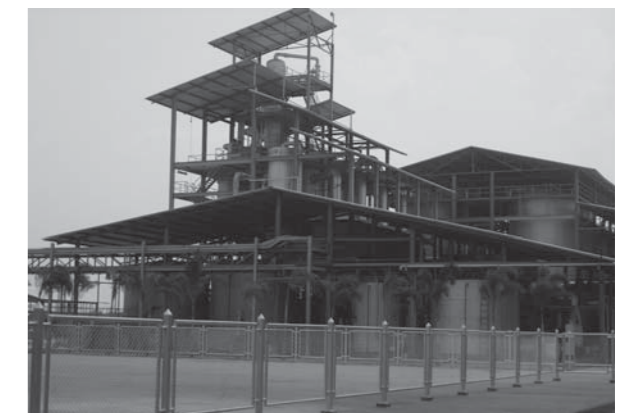
図7 濃縮・蒸留・脱水設備 Fig.7 Evaporation, distillation and dehydration plant
