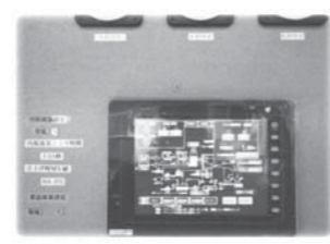
図6 現場盤にある操作TP Fig.6 Touch panel for operating on the local control panel
