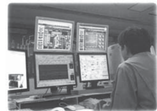
図2 汎用PC(水処理監視室) Fig.2 Monitoring by computer in the monitoring room
