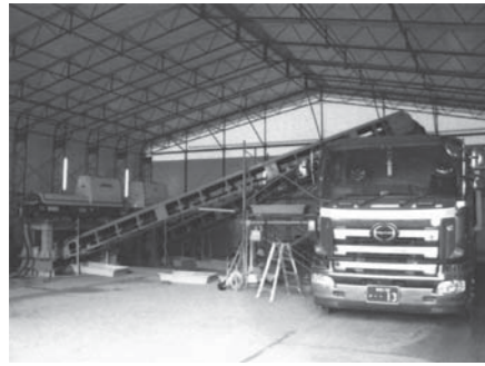
図5 仮設脱水設備 全景 Fig.5 Full view of the temporary dewatering machine
