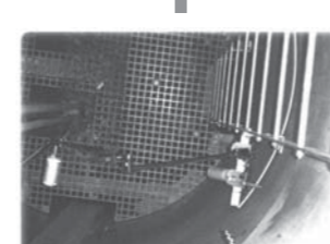
図11 ②マンホールP内の監視 Fig.11 Monitoring for manhole pump
