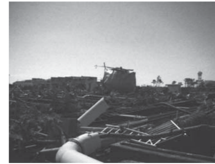
図1 震災後の被害状況(最初沈殿池周り) Fig.1 Damage around the primary sedimentation tank after the Great East Japan Earthquake
