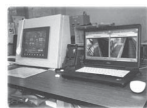
図7 汚泥処理監視室内の遠隔操作TPと映像用PC Fig.7 Touch panel for remote operating and computer for monitoring
