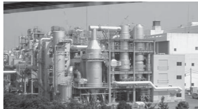
図4 流動炉概観 Fig.4 Overview of fluidized bed incineration plant
