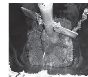
図1-6 設置前(約1ヶ月)凝集混和槽 Fig.1-6 Month before augmentation - coagulation mixing tank
