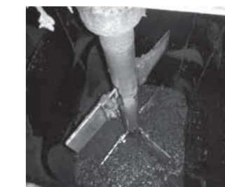
図1-7 設置2ヶ月後 凝集混和槽 Fig.1-7 2 Months after augmentation - coagulation mixing tank
