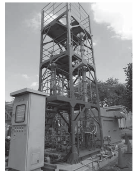
図6 消化ガス精製装置 Fig.6 Digestion gas refinement system
