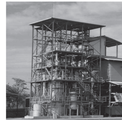
図1 実証設備の外観 Fig.1 Photo of demonstration plant
