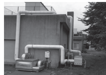
図7 需要家設備 Fig.7 Customer facility
