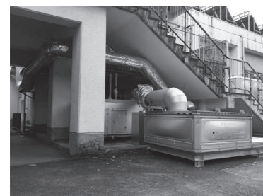
図10 需要家設備 Fig.10 Customer facility
