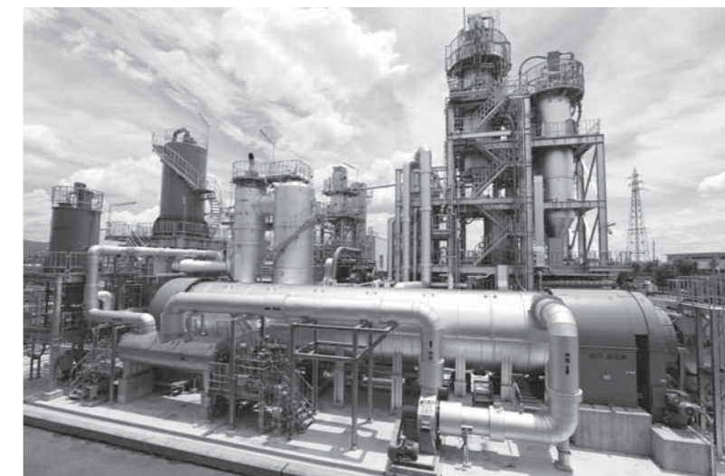
図4 燃料化施設外観 Fig.4 External view of sewage sludge fuel conversion facility.
