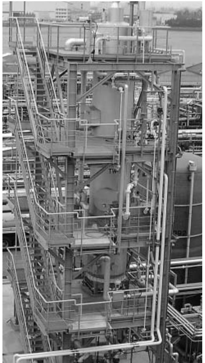
図 6 VOC 除去設備 Fig.6 VOC removal plant system
