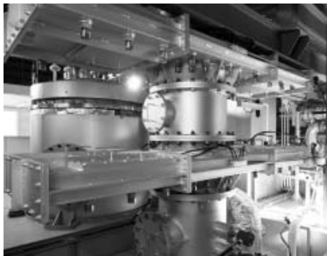
図4 ガス化炉外観 Fig.4 External view of gasifier
