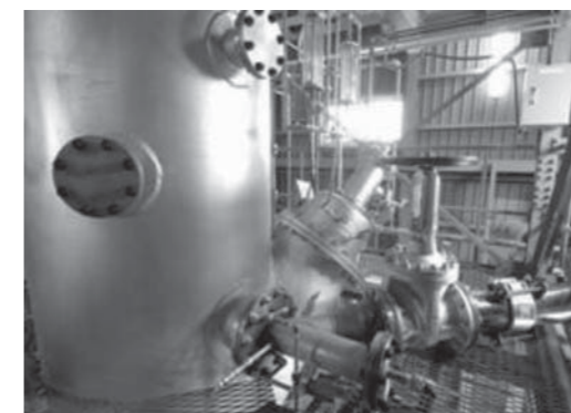
図6 過給式流動炉(汚泥投入部) Fig.6 Photo of Fluidized Bed Incinerator with turbocharger
