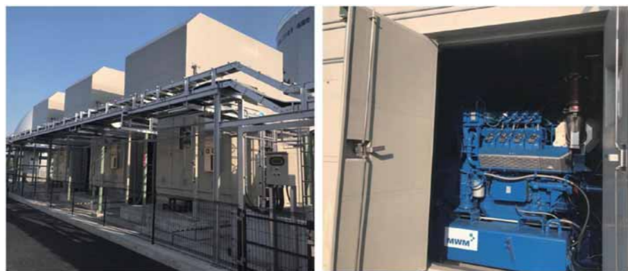
図4 消化ガス発電機 Fig.4 Appearance of digestion gas power generator
