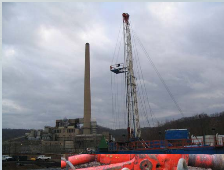
Deep Well Rig
