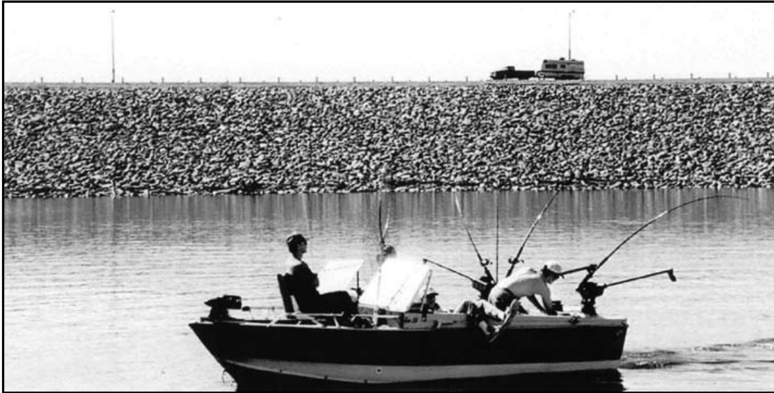
Figure 6-29: The riprap on the upstream face of Garrison Dam. Source David P. Billington.
