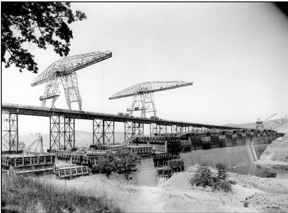
Figure 7-15: Friant Dam under construction showing the trestle and crane construction system used to deliver concrete and form work used in building the dam. Source: Donald C. Jackson collection, courtesy of John Snyder.
