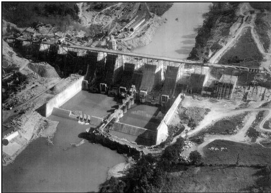
Figure 8-4: The downstream face of Tygart Dam during construction. Source: Records of the U.S. Army Corps of Engineers, Record Group 77, National Archives and Records Administration, College Park, Maryland.
