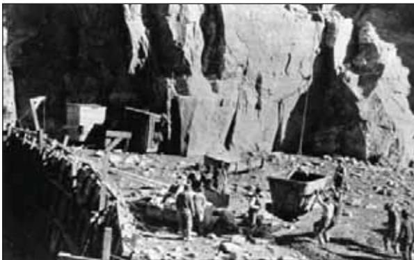
1.5. Construction at Buffalo Bill Dam, Wyoming. Note wooden forms at downstream face and plum stones protruding from previous lift.
