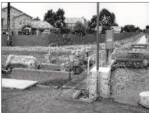
10.9. The SCADA system on the Salt River Project controls this canal control structure. Courtesy of the Salt River Project.
