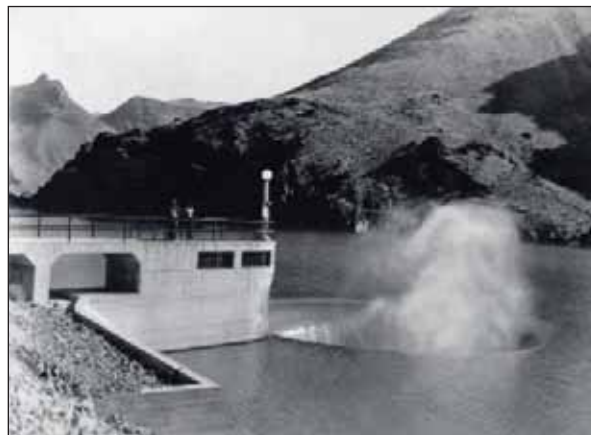
1.20. Owyhee Dam, Oregon. Spillway “Burp” (unstable flow condition, sometimes referred to as “blow-back”).
