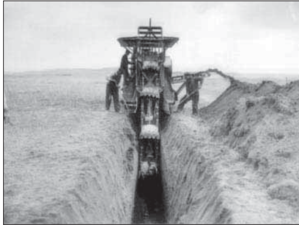
4.2. An Austin trencher digging a drain on the North Platte Project in 1917.
