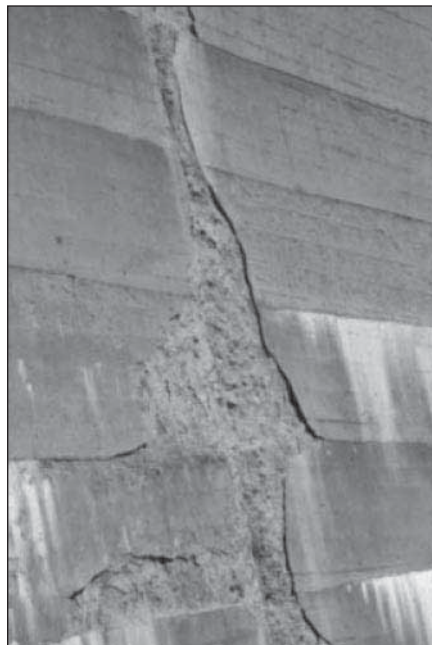
1.36. Freeze-thaw damage on downstream face of Deadwood Dam, Idaho. (Note that damage is near contraction joint due to leakage.)
