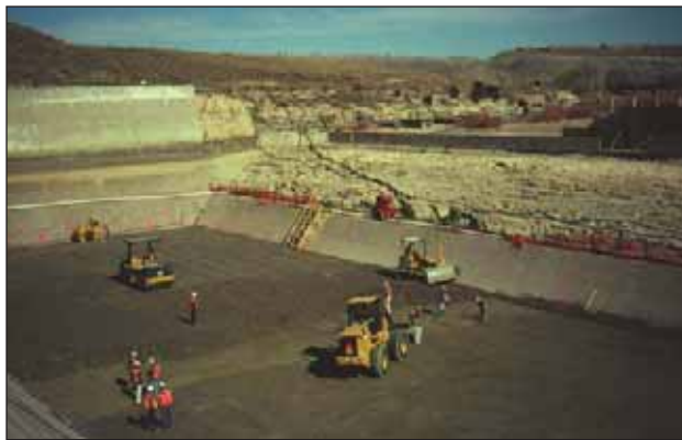
1.54. RCC placement, spreading, and compaction operations in the spillway pool, Pueblo Dam, Colorado.
