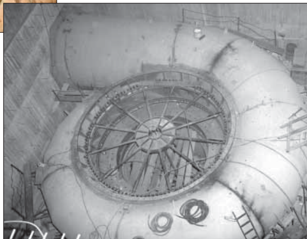
31.5. The scroll case in unit 5 of the Glen Canyon Powerhouse during installation in 1963.
