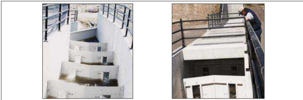
6.10. Marble Bluff Dam Fishway exit Ladder.
