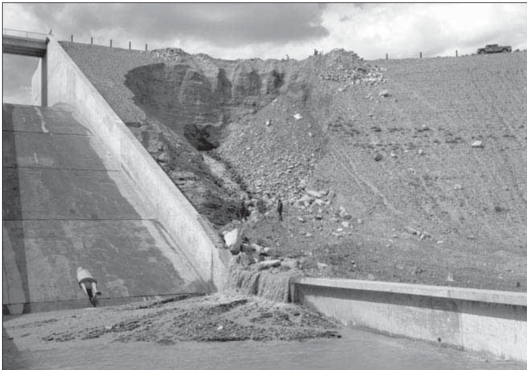
2.12. Fontenelle Dam: Large sinkhole on downstream slope.
