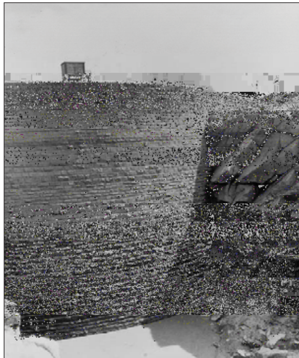
8.5. Upstream face of Pathfinder Dam on the North Platte River near Casper, Wyoming, is a masonry arch and cantilever section. Source: Bureau of Reclamation.
