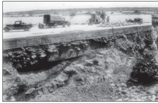
32.5. CCC men working on McMillan Spillway No. 2, Carlsbad Project, New Mexico, in 1938.
