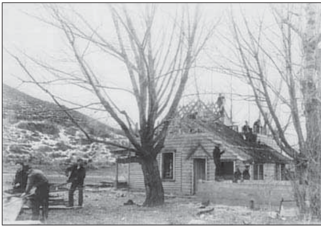
17.3. This 1940 photograph by Ellis Armstrong, later a Commissioner of Reclamation, shows CCC forces dismantling the Atwood house in the Deer Creek Reservoir area near Charleston on the Provo River Project.
