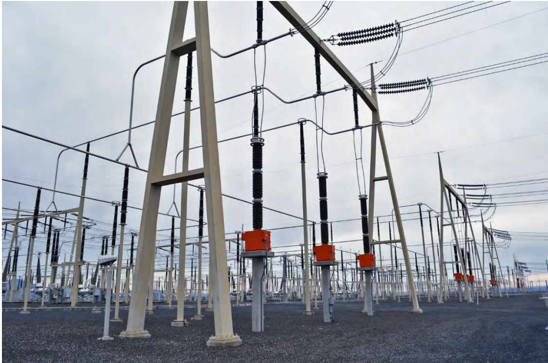
500kV Switchyard, Columbia Basin Project, Pacific Northwest Region.
