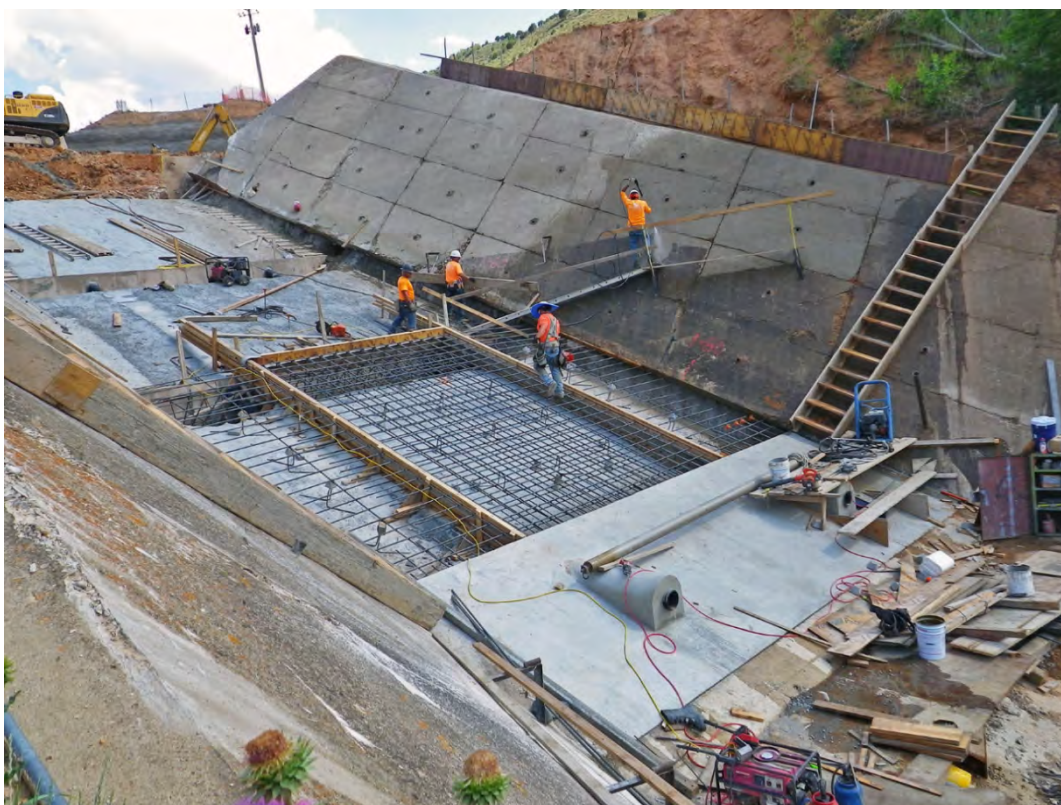
Echo Dam Safety of Dams Modification, Weber Basin Project, Upper Colorado Region.
