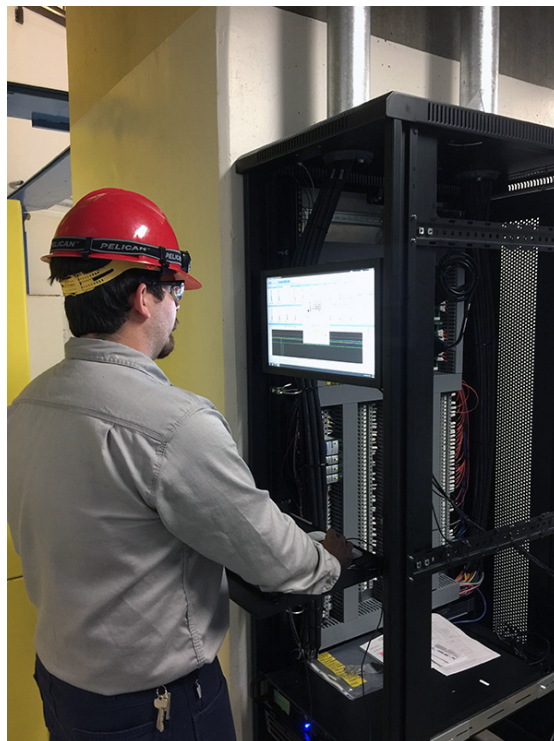
Collecting Generator Monitoring Data using Reclamation Developed MCM System.
