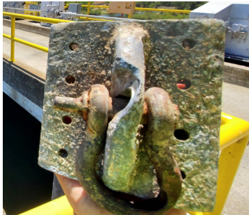
Conventionally-manufactured log boom anchor at Nimbus Dam, California.
