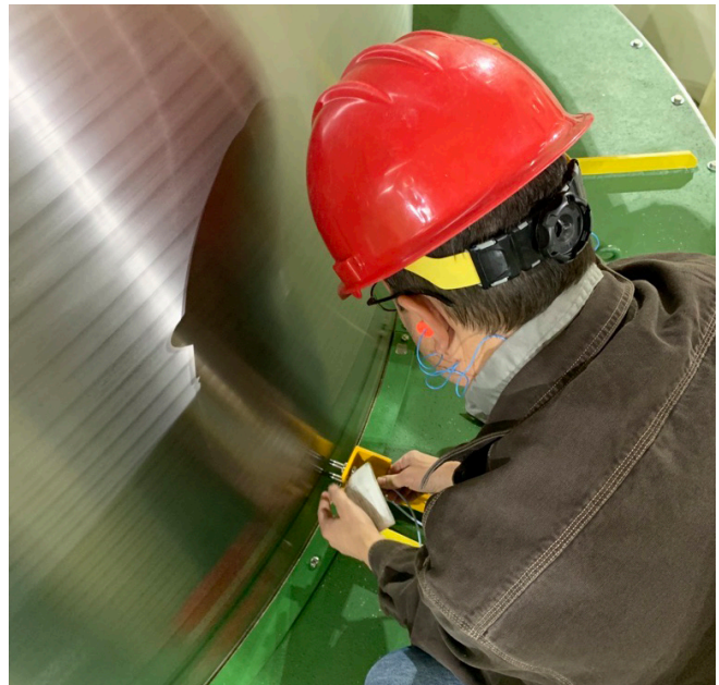
Adjustment of Proximity Probes at the Turbine Guide Bearing used for Vibration Monitoring.
