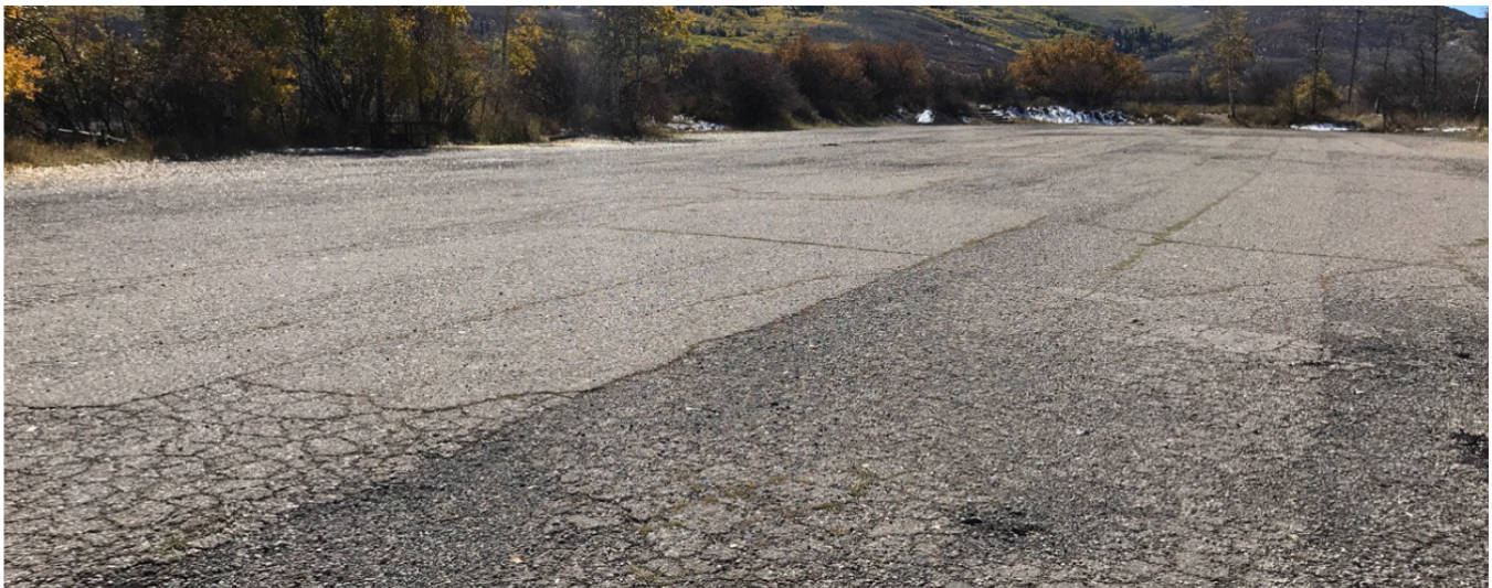
Example of pavement distress documented during a parking lot condition assessment.
