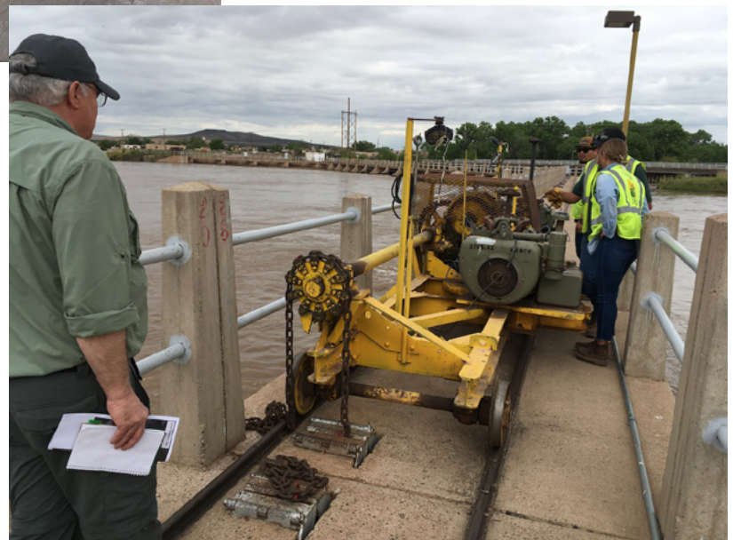
The river gates of the Isleta Diversion Dam are still operated manually with a "mule" and team of dam tenders. (Reclamation, C. Gombert, May 2023)
