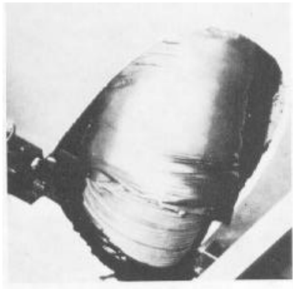
A fire-resistant ceiling is not effective if an architect or a workman allows wide holes for a pipe to pass through.
