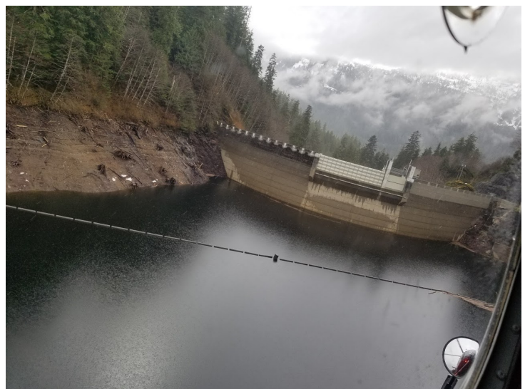
Swan Lake reservoir showing record low water. Photo courtesy of Southeast Alaska Power Agency (SEAPA)
