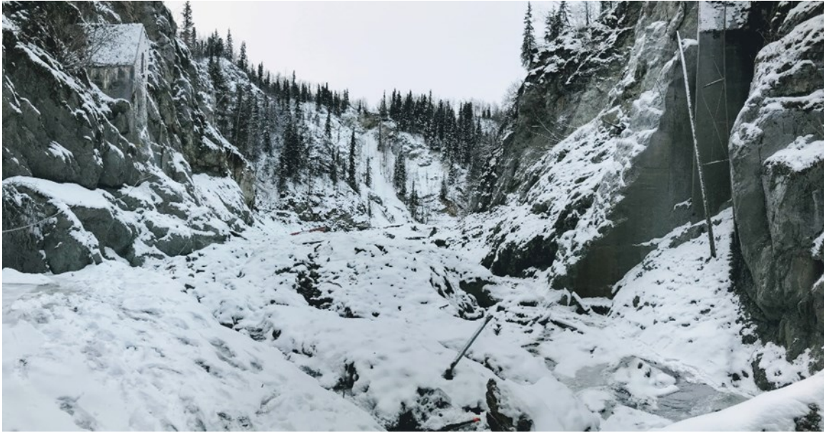
Photo: Looking upstream at remnants of the lower Eklutna Dam. Demolition of this concrete arch dam is ongoing. Credit: Crane Johnson, APRFC/NWS.
