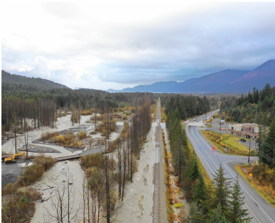
Figure 10: heavy equipment is helping preserve this bridge near Seward by removing gravel from the streambed as it's washed down by heavy rain. Photo courtesy of Alaska DOT&PF.
