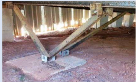
Figure 2: Example of pan anchorage for a pier-block foundation residential construction. From Analysis of Manufactured Home Vulnerability in Extreme Winds , Davis, B. M., 2020.
