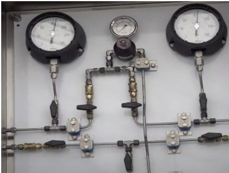
Figure C-2: Hydrogen Line Pressure Gauge (Varies per site)
