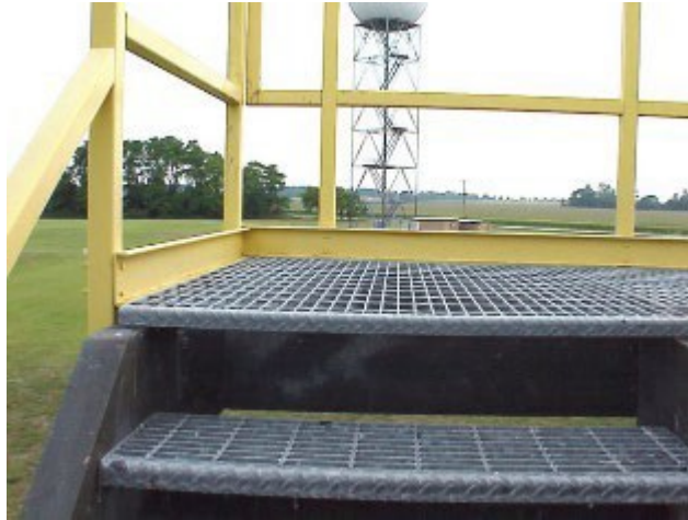
Figure K-13: Foot Plate at Top of Stairs
