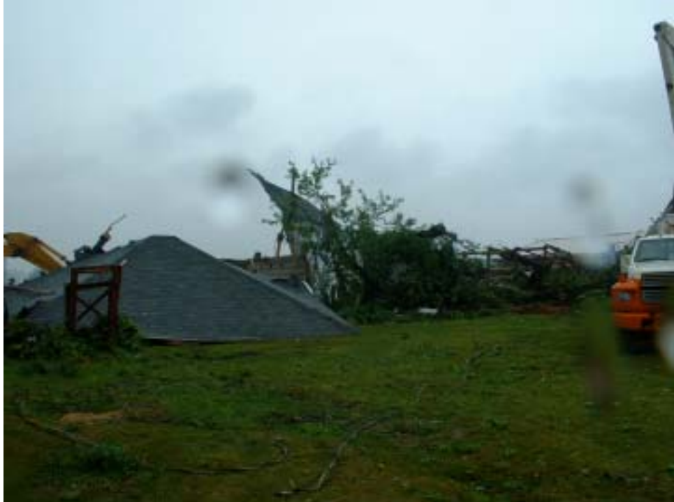
Looking west toward destroyed garage
