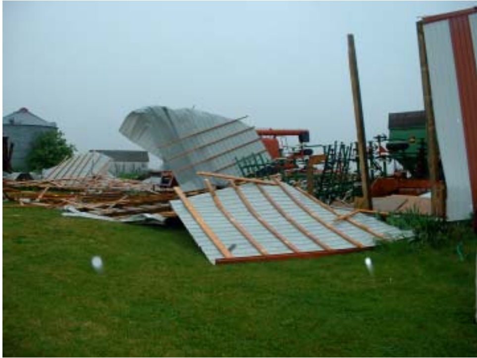
Southwest wind blew down outbuilding, looking southeast
