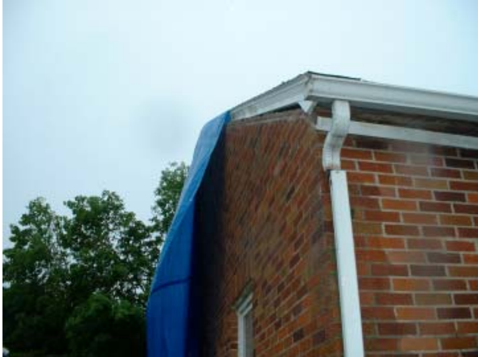
Roof of house displaced
