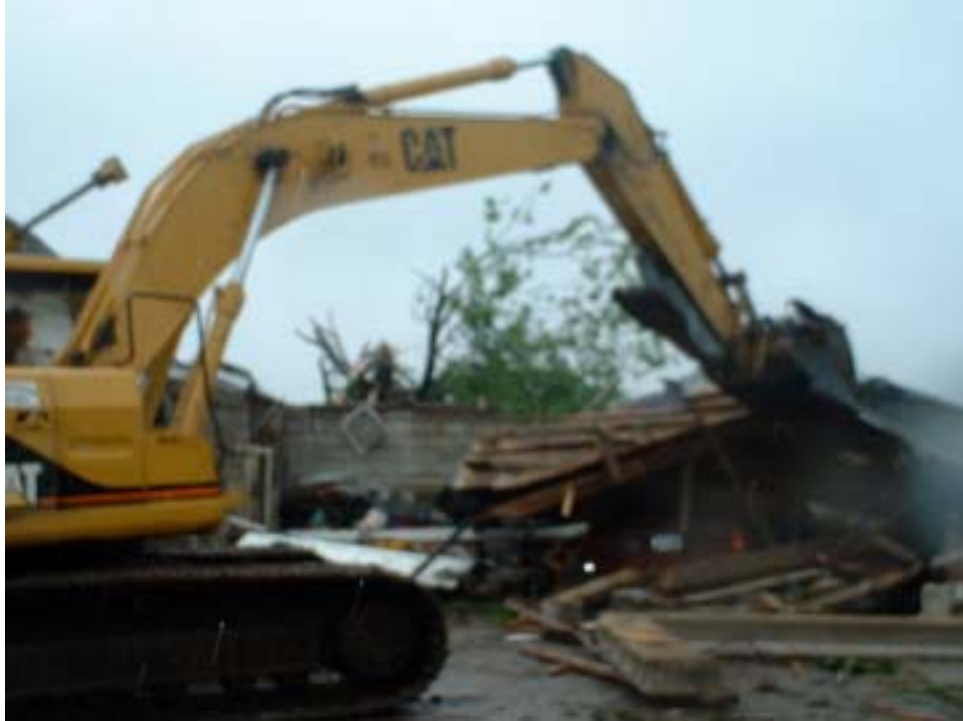
Looking north to destroyed garage
