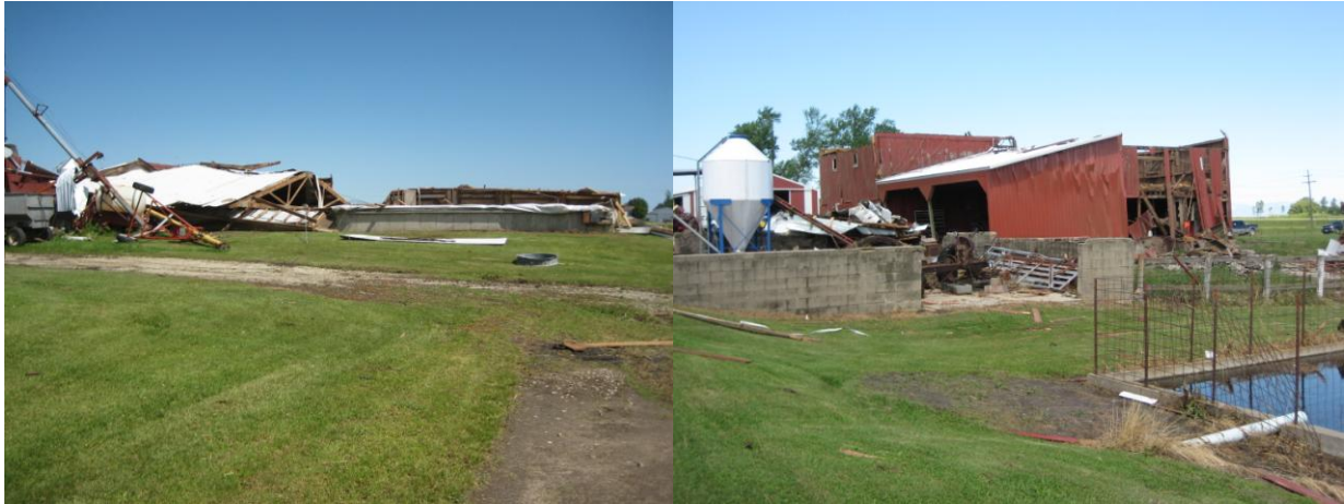
Barn damage to barns and outbuildings at Point 1 which was caused by straight-line winds of between 85 and 90 mph
