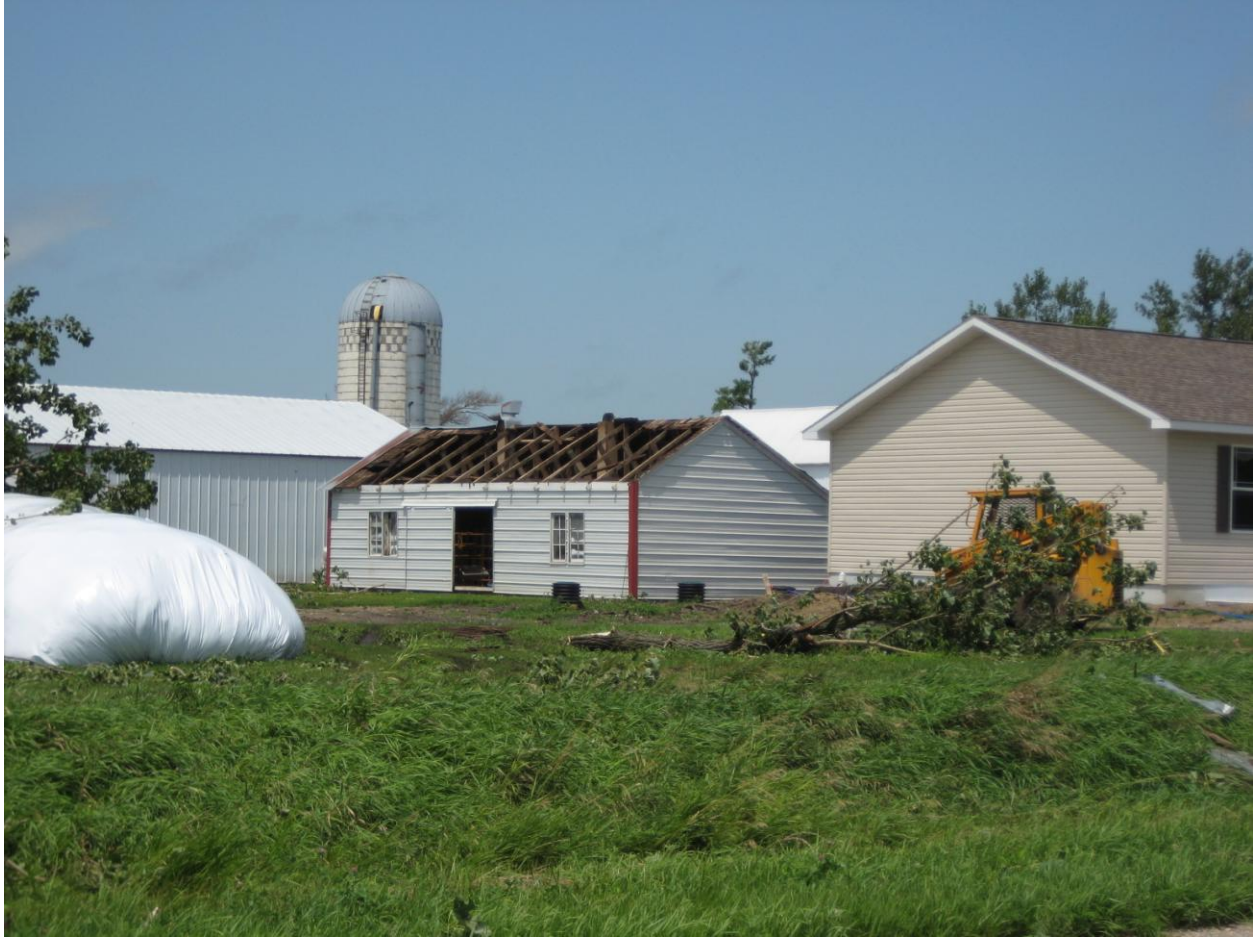
Figure 3. A building with roof damage near on the south end of Pocahontas.
