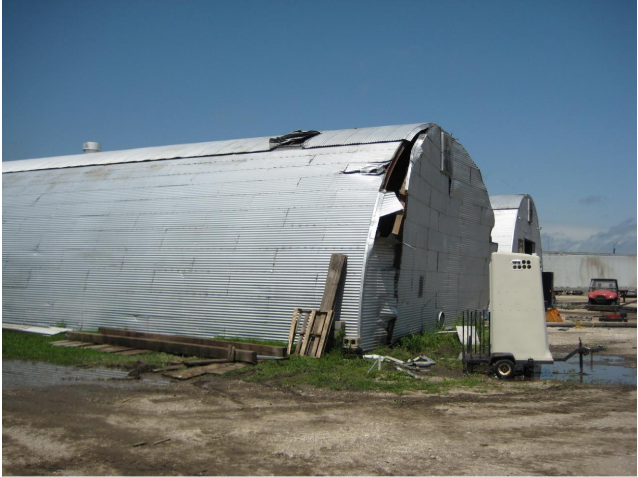
Figure 6. The end of this Quonset hut was blown out and was found laying flat on the ground. Workers had attempted to place the wall back in the vertical position by the time the photo was taken.
