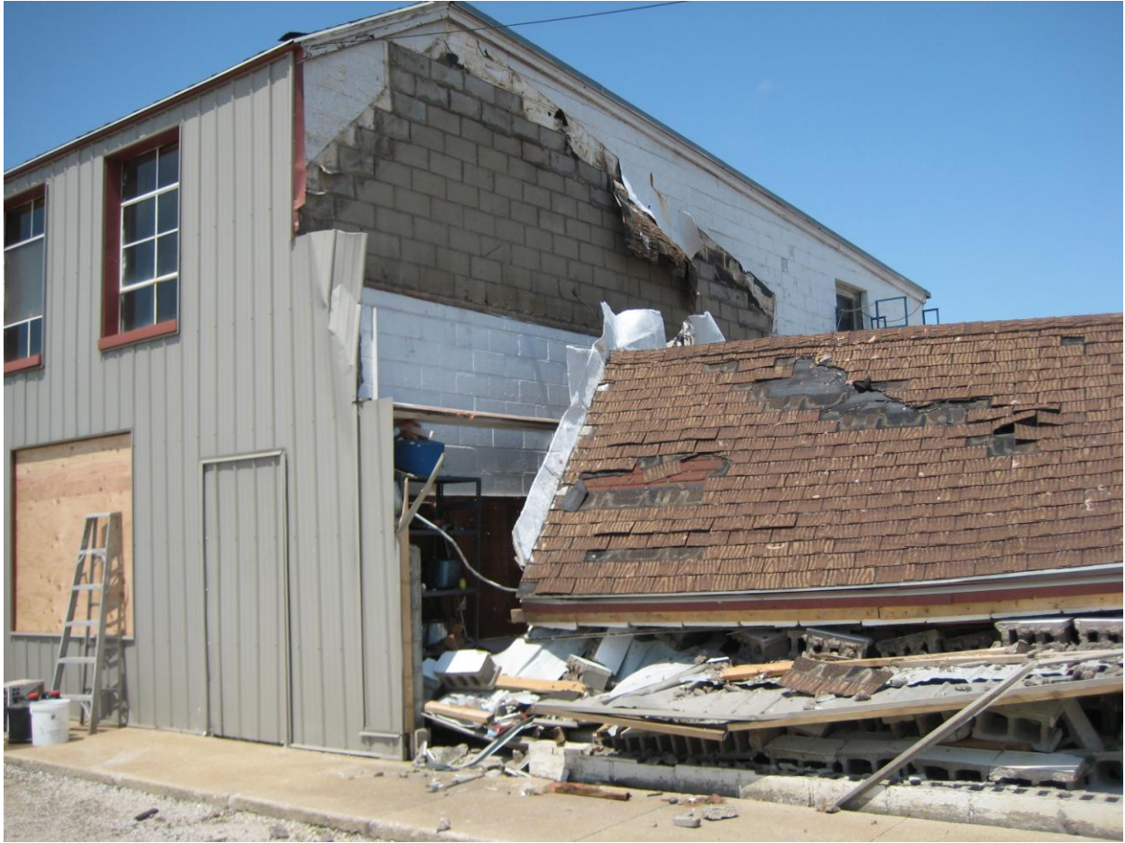
Figure 7. The cinder block wall of this building collapsed and the roof was torn off the side of the parent building in eastern Pocahontas.
