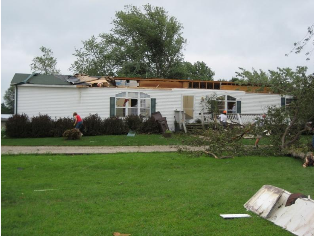
Figure 3. Damage to a house north of West Euclid Avenue.
