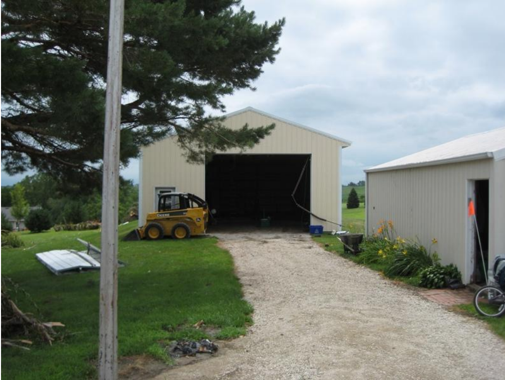
Figure 8. Damage to a garage belonging to a house south of Jersey Street.
