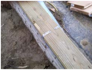
Anchored sill plate. At same site of house that slid off its foundation. Photo by NWS Des Moines, Iowa.
