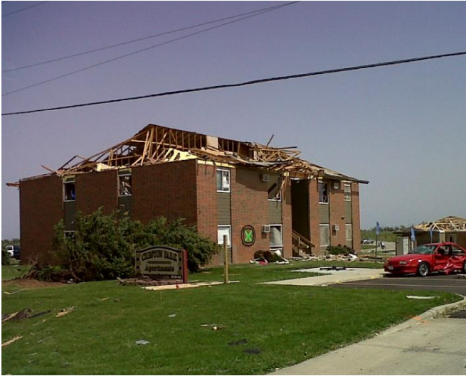
An apartment building sustained roof damage. Cars in the parking lot were dented and damaged.
