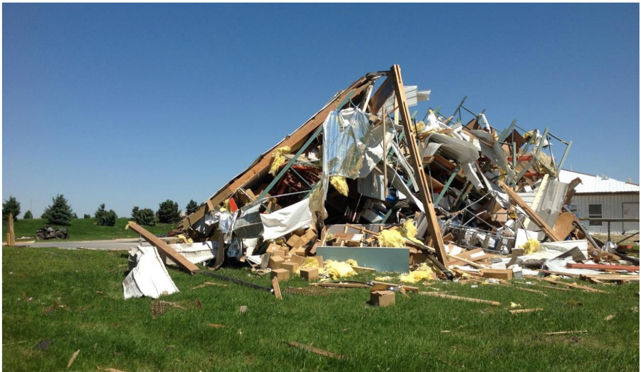
A warehouse was destroyed and partially swept from its foundation on the north side of Belmond.
