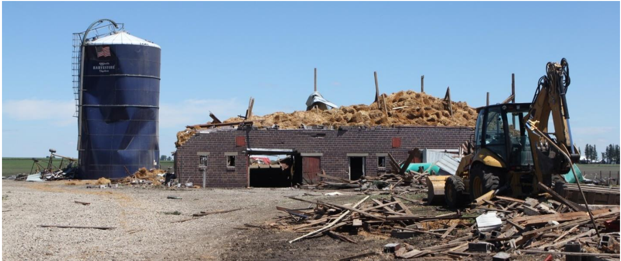
A destroyed barn near the beginning of the track north of Alexander. Photo by Tim McCleary
