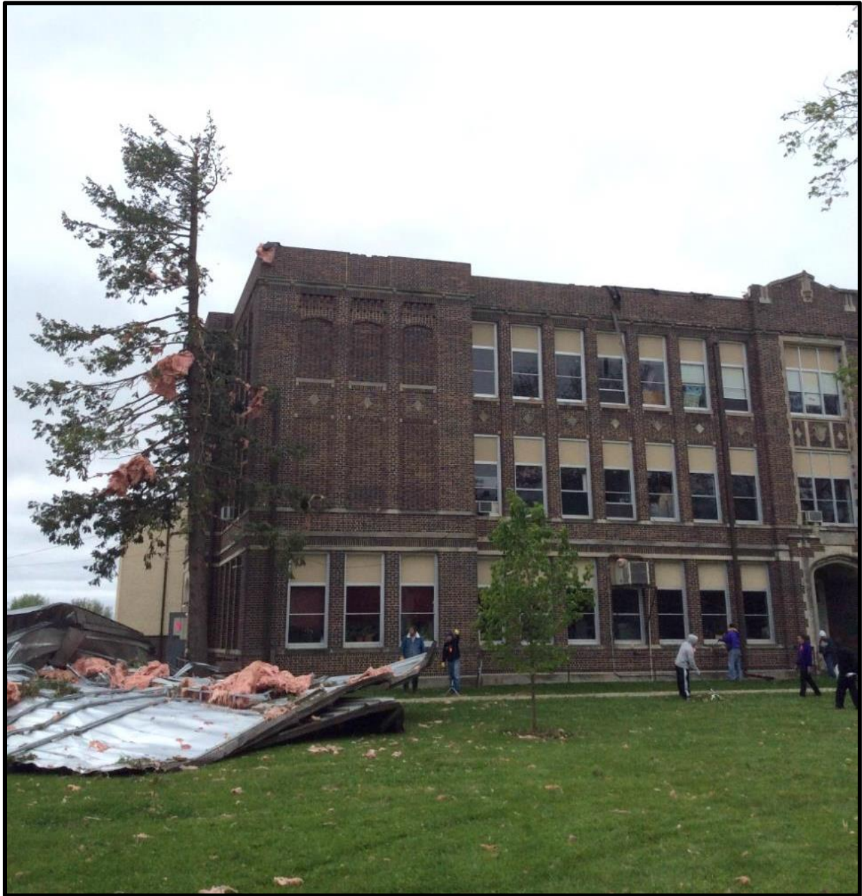
The roof was torn off the high school in Lake City. The tornado was rated a higher-end EF-1 with a maximum wind speed of 100 mph at this location
