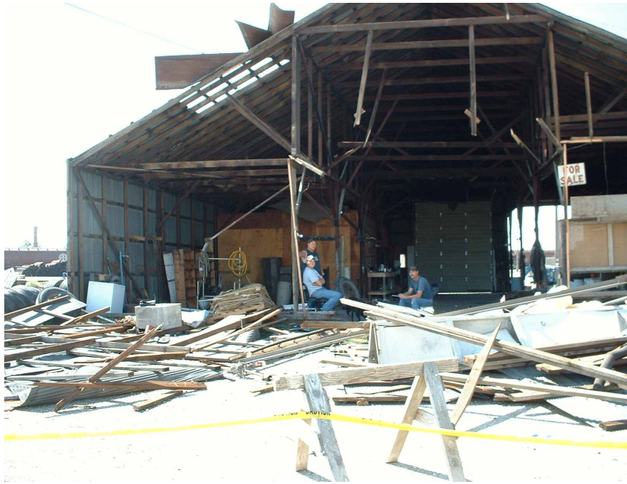
Metal building with major damage. Wind entered building from the back door and blew the front wall out. Building was located near downtown Creston.
