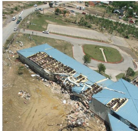
School Roof Damage
