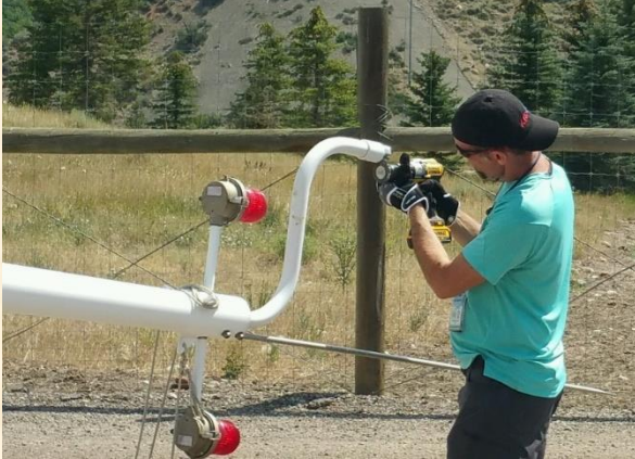
Image 1: ET Mike Martinez using a cordless drill to sand the edges of the alignment collar of an ASOS so the new IFWS will fit properly. Photo credit: NWS.
