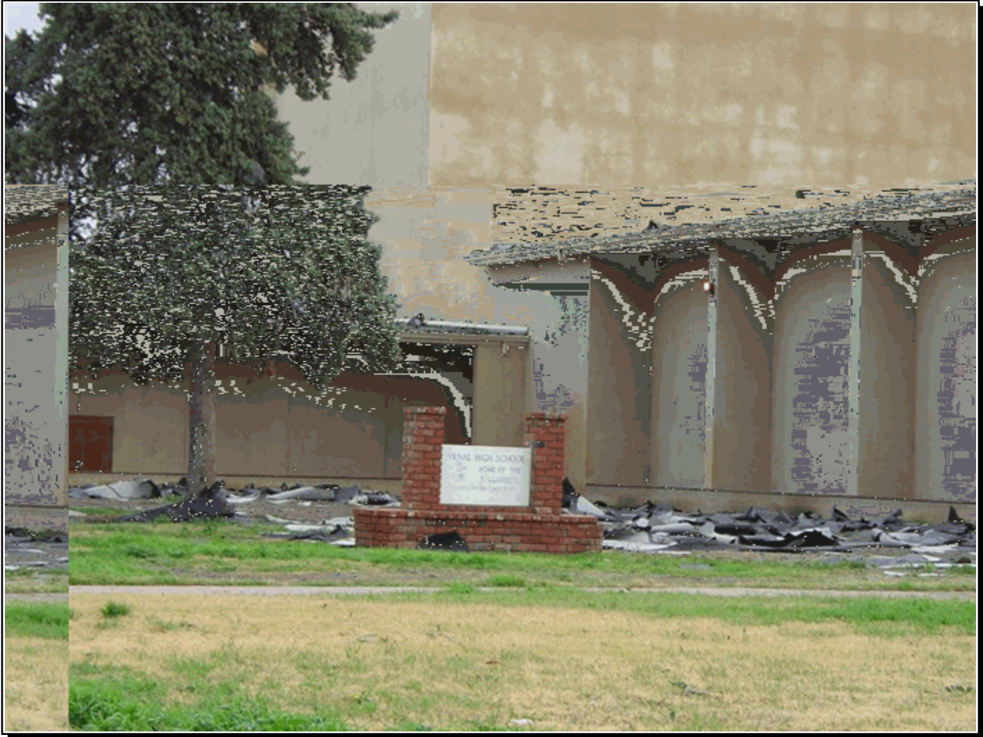
Widespread roof damage at Avenal High School. High winds were caused by a combination of strong large-scale winds and the local development of a mountain rotor cloud. Peak winds estimated at 70-75 mph. Photo courtesy CA Office of Emergency Services.
